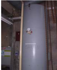
OAK-451 1. Tank, Water Well Pressure
