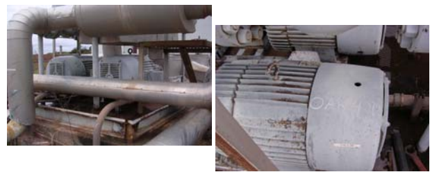
OAK-426 A 1. Pump and Motor Assembly
