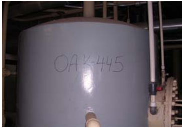
OAK-445 1. Tank, Miscellaneous Drain
