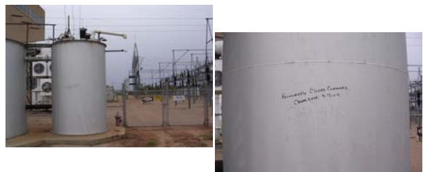
OAK-418 1. Tank, Storage
