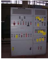
OAK-407 1. Switchgear Panel, Breakers, 2 Sections
