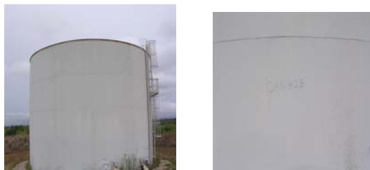
OAK-428 1. Tank, Fuel Oil Storage
