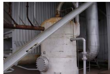
OAK-422 1. Pressurized Vessel
