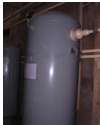
OAK-449 1. Tank, Air Receiver (Station Air)
