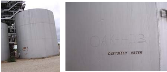
OAK-423 1. Tank, Distilled Water
