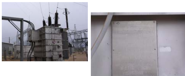
OAK-419 1. Transformer, Power Transformer
