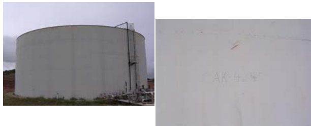
OAK-425 1. Tank, No 4 Fuel Oil Storage
