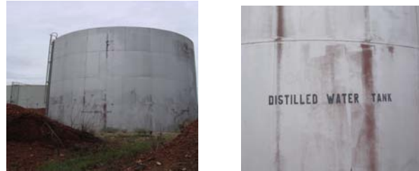
OAK-427 1. Tank, Distilled Water Storage
