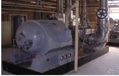
PEC-031 1. Pump, Centrifugal
