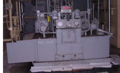
PEC-028 1. Hydrolic Fluid Power Unit
