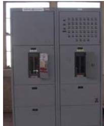
PEC-009 1. Panel, Switchgear - 2 Sections
