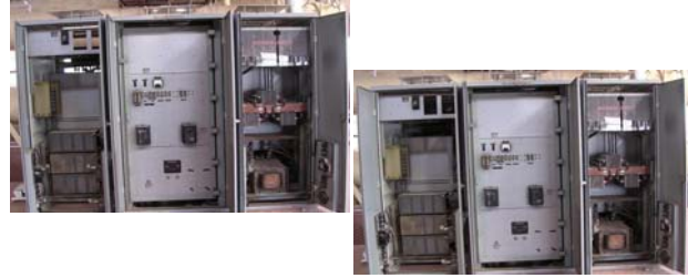
PEC-008 1. Panel, Switchgear - 3 Sections
