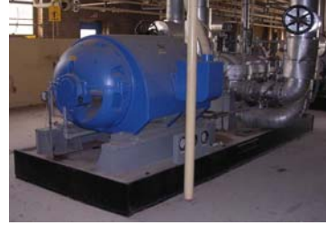
PEC-032 1. Pump, Centrifugal
