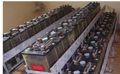
PEC-076 2. Battery Chargers / Rectifiers
