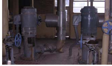
PEC-024 1. Pump, Centrifugal - Vertical
