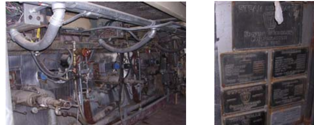
PEC-010 1. Boiler, Steam Generator 3 Burner
