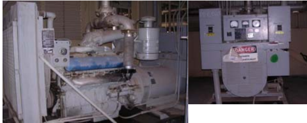
PEC-025 1. Generator Set
