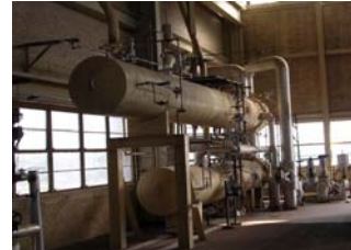
PEC-004 1. Exchanger Heat
