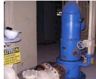
PEC-036 1. Pump, Centrifugal - Vertical
