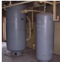
PEC-033 1. Tank, Air Receiver
