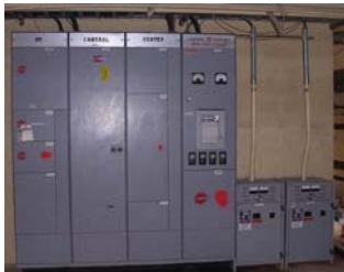
PEC-075 1. Motor Control Center - MCC DC
