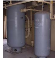
PEC-034 1. Tank, Air Receiver
