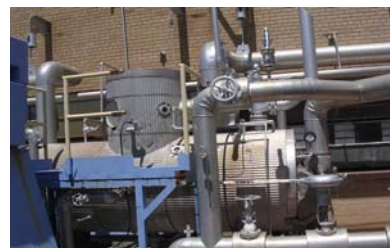
PEC-014 1. Exchanger, Heat - Evaporator
