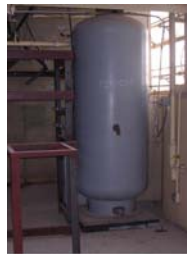
PEC-035 1. Tank, Air Receiver
