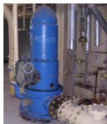
PEC-037 1. Pump, Centrifugal - Condensate Pump
