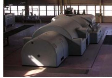
PEC-002 1. Steam Engine – Generator Unit (#5)
