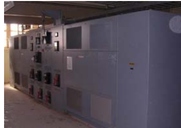
PEC-074 1. Switchgear Panel - Control
