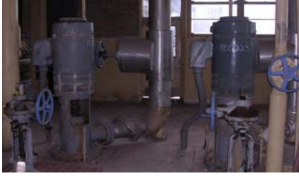
PEC-023 1. Pump, Centrifugal - Vertical
