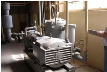
PEC-029 1. Compressor, Air - Unit #1
