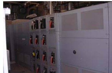
PEC-012 1. Panel - Switchgear with Transformer and 12 Panels
