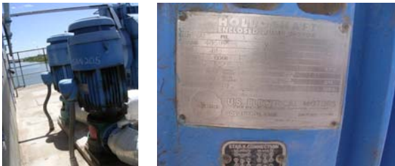
SAN-205B Pump & Motor Assembly
