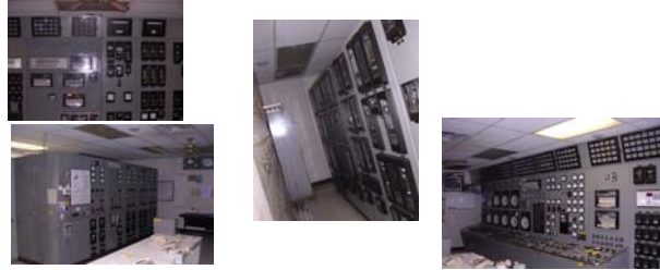
SAN-215 Control Room
