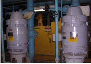
SAN-207A Pump & Motor Unit
