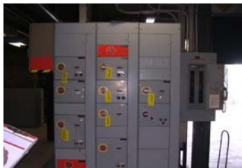
SAN-267 Switchboard Panel
