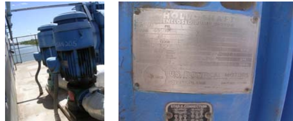
SAN-205A Pump & Motor Assembly
