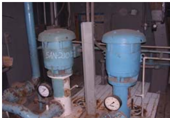
SAN-210A Pump & Motor Assembly
