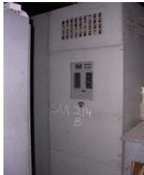
SAN-214B Panel, Breaker
