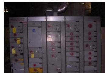
SAN-212 Motor Control Center- MCC
