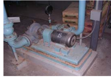
SAN-262B Pump & Motor Assembly
