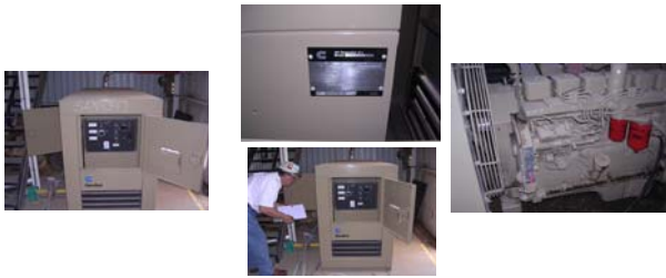
SAN-247 Generator Set
