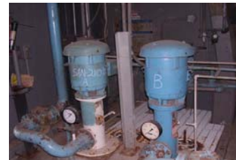
SAN-210B Pump & Motor Assembly
