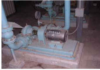
SAN-262A Pump & Motor Assembly
