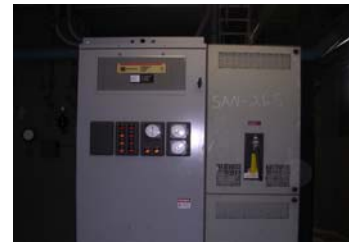
SAN-268 Switchboard Panel
